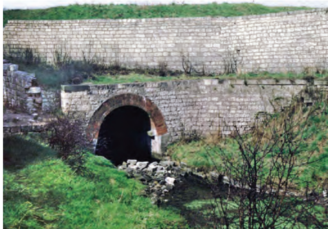
The eastern portal of Norwood tunnel in the early 1960s, shortly before the portals were sealed by British Waterways
